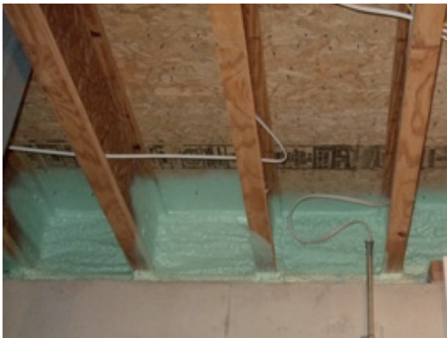
FIGURE 12. Closed-cell SPF insulation at the foundation-framing area
